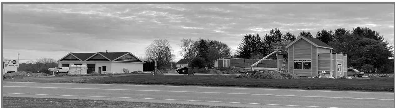
Newport's construction zone in November: Newport Carwash on left, Aroma Joe's on right. Opening soon?
